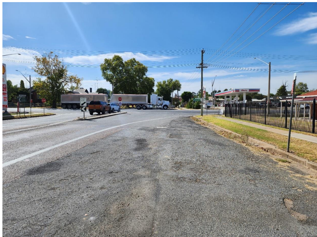
Fig 2: Intersection looking east from Audley St (noting slope of roadway and distance to footpath)
