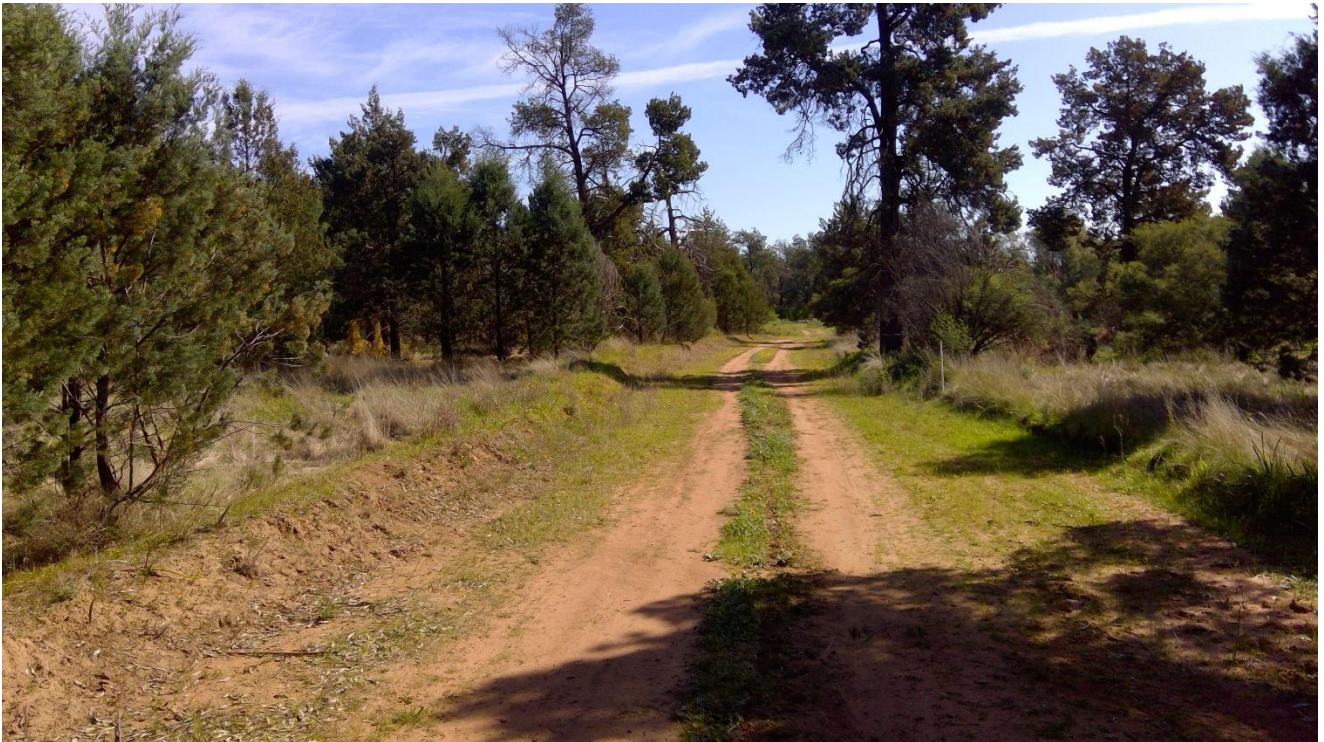
Figure 16: Current state of Hartnett Rd to be upgraded to public access road standards – 5.5m wide carriageway, 2wd all weather surface.
