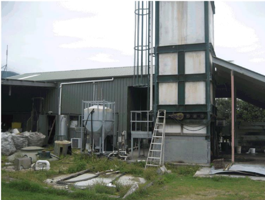
Vertical Composting Unit
