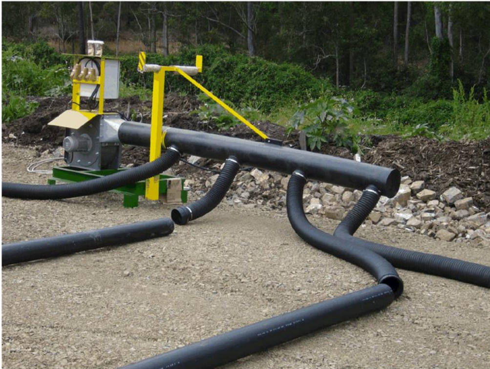
MAF blower, manifold and air distribution pipes
