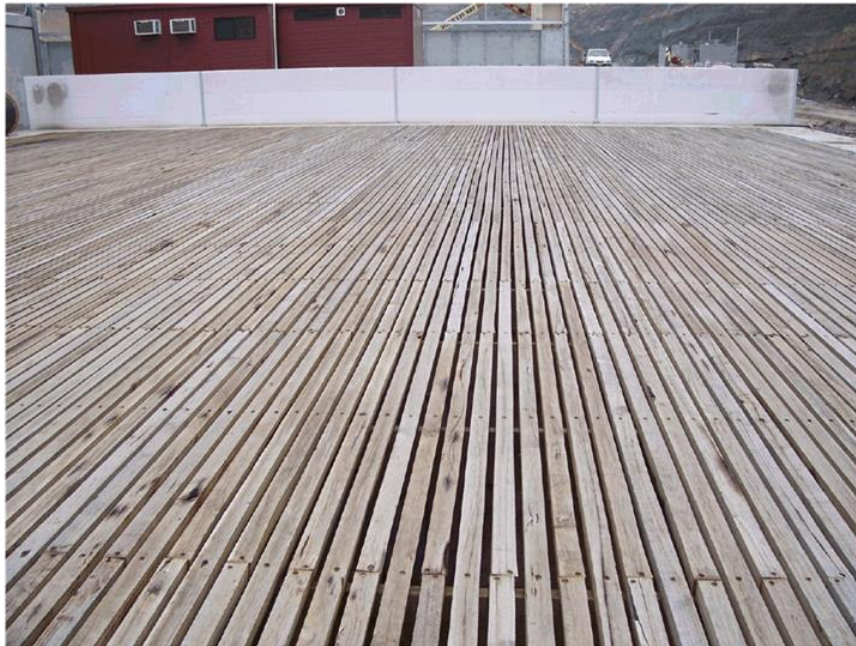
Bio filter before filter material is added
